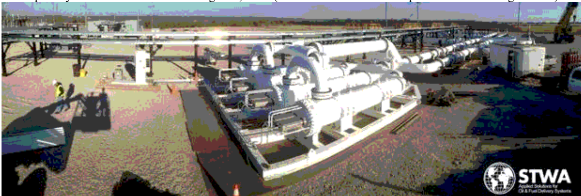
4-Unit AOT installed on TransCanada's Keystone Pipeline, cumulative capacity of 600,000 barrels per day.
