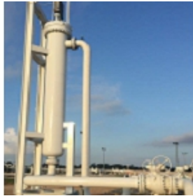
Single-Unit AOT installed on KMCC's pipeline, capacity of 200,000 BBL/Day.
